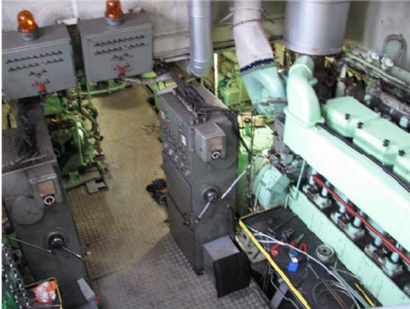
Figure 4.3 Current Skoda main engine and engine room of Dunaföldvár
