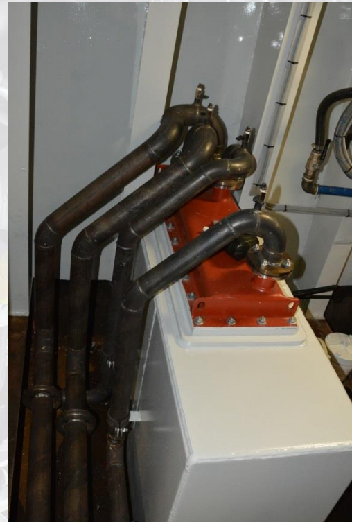
New box cooler
