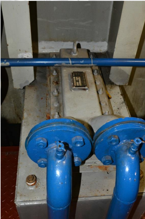
Old box cooler
