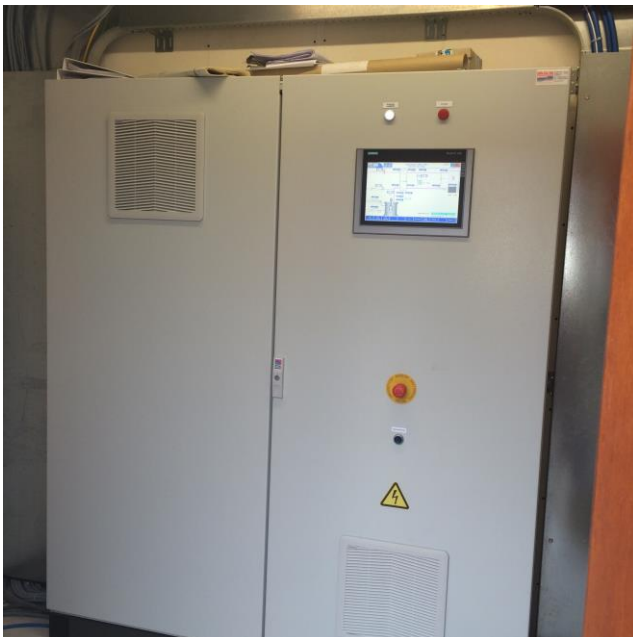
Picture: Control cabinet incl. HMI
